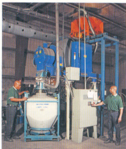
An operator (left) positions a bulk drum under the blender's discharge, while another operator (right) calls up a preprogrammed recipe on the blender's control panel.
